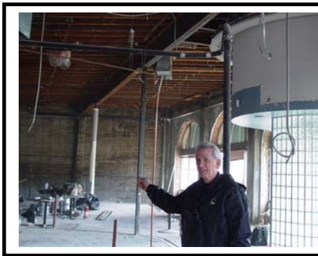
Stu Freeman points to the restoration work which will become the home of a new restaurant and bakery soon.
